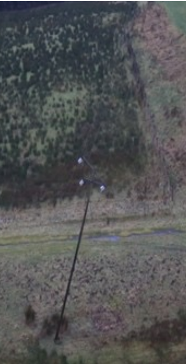
Figure 21: Leaning pole on 38kV network (Cathleen Falls 38kV)
