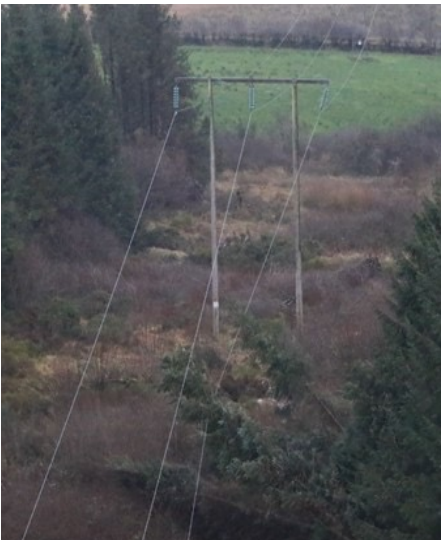
Figure 18: Forestry Fault, Cavan (Rathrussan – Shankil 110kV line)
