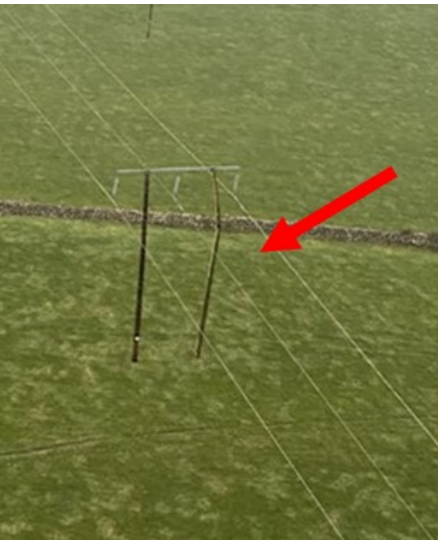
Figure 17: Broken Pole, Galway (Cashla Cloon 110kV line)
