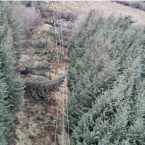
Figure 23: Forestry impacting fault on 38kV network (Loughrea – Sonnagh 38kV)
