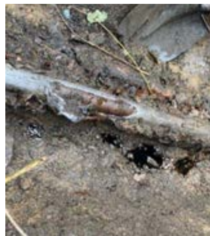
Damage to fluid-filled cable caused by house building contractor
