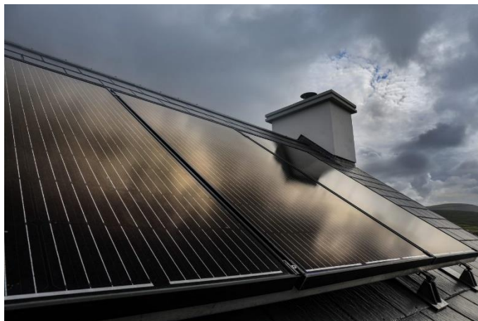
FIGURE 6 SOLAR PV ARRAY
