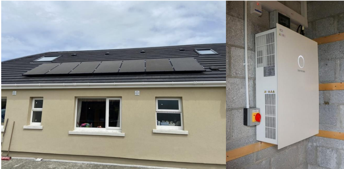
FIGURE 4 SONNENBATTERIE 9.53 HYBRID BATTERY & SOLAR INSTALLATION
