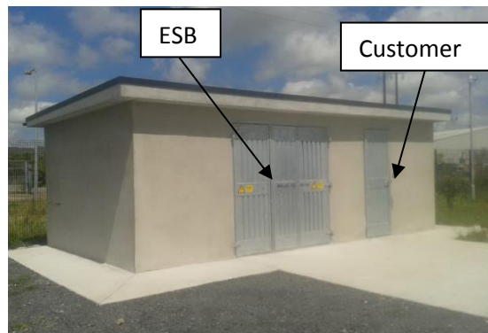
Fig. 2: Freestanding MV substation adjoining a customer's switchroom.
