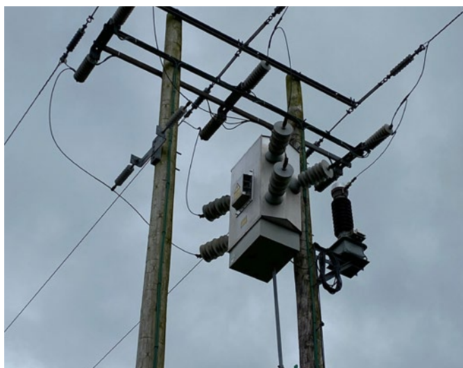
38kv remotely controlled switch
