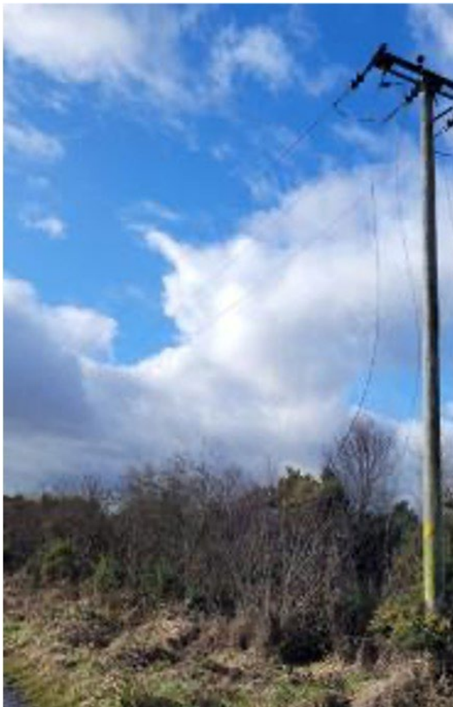
Third party damage causing grounded electricity line
