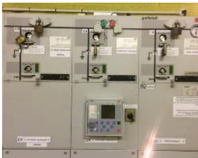
MV urban switch automation
