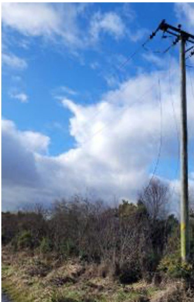
Third party damage causing grounded electricity line
