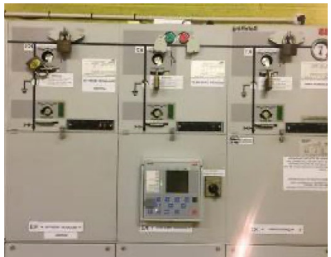
MV urban switch automation
