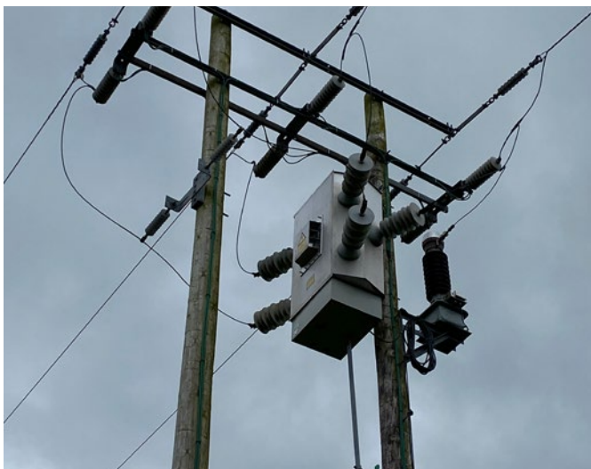
38kv remotely controlled switch
