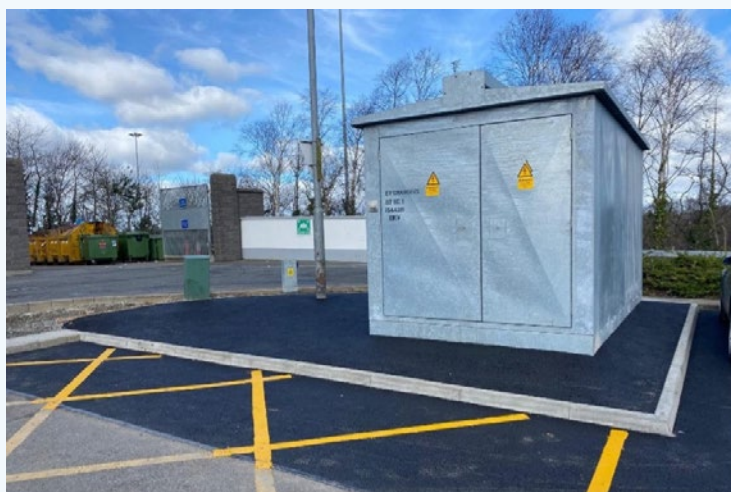
(a) EV Charging Hub module at Blanchardstown
