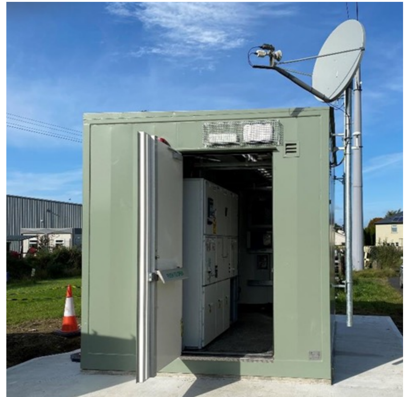
Figure 3: EGIP Modular Standard Substation
