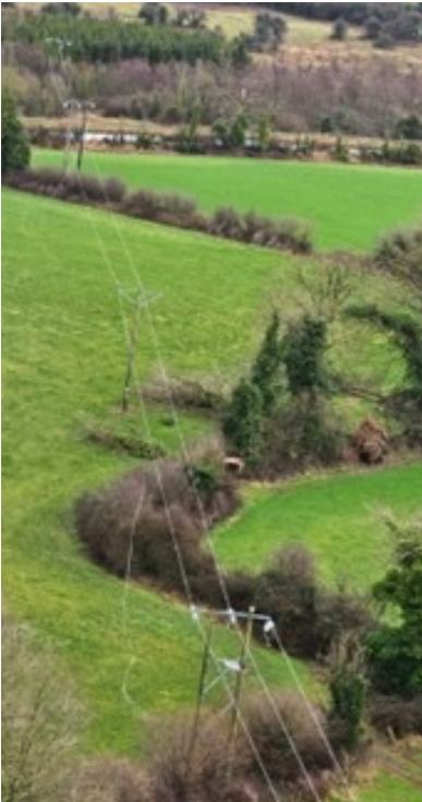
Figure 20: Broken Conductor on 38kV network (Aghamore – Ballymahon 38Kv)
