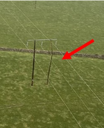
Figure 17: Broken Pole, Galway (Cashla Cloon 110kV line)
