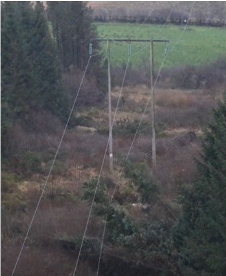
Figure 18: Forestry Fault, Cavan (Rathrussan - Shankil 110kV line)
