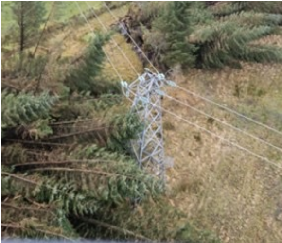
Figure 22: Forestry impacting fault on 38kV network (Castlerea – Raheen Bar 38kV)
