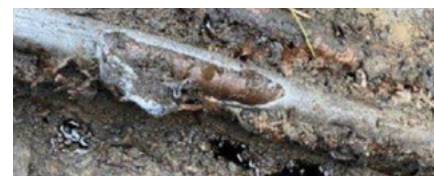
Damage to fluid-filled cable caused by house building contractor
