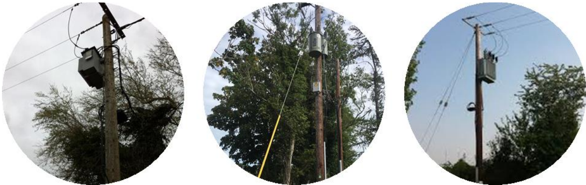
FIGURE 11. POLE MOUNTED TRANSFORMERS
