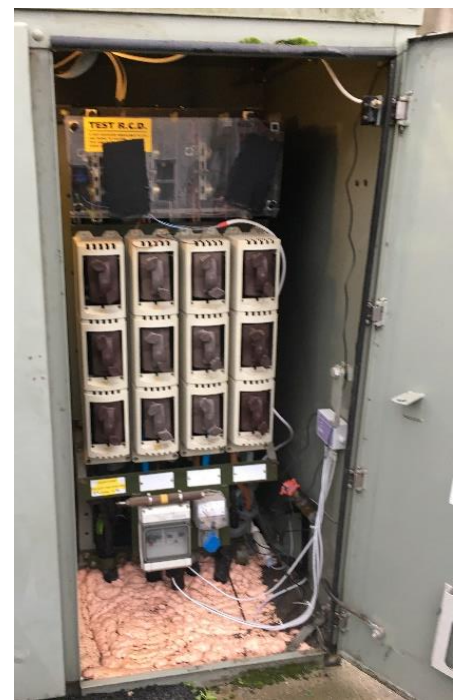
Figure 2 - MV/LV substation with monitoring device installed
