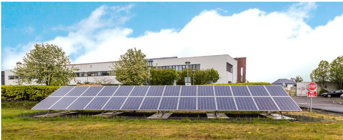
Figure 7. PV Installation at ESB Networks Training Centre, Portlaoise
