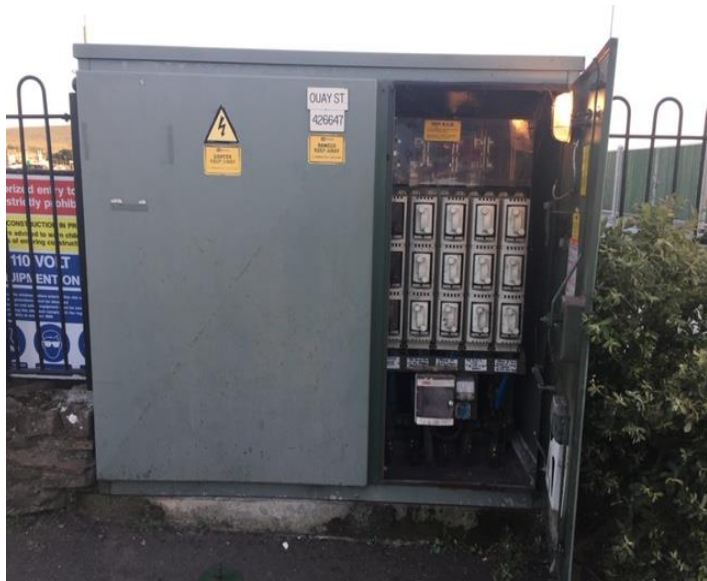
FIGURE 4. GROUND MOUNTED SUBSTATIONS
