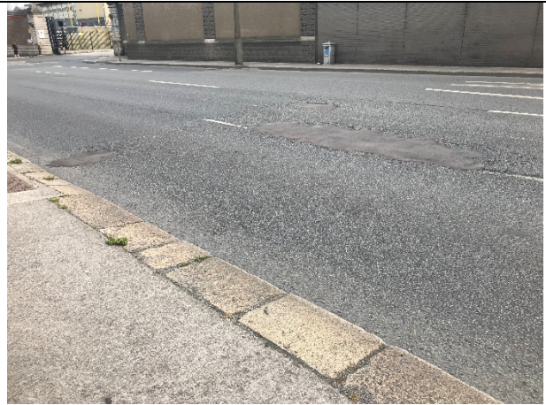
10-04 – Road surfacing in generally good condition on Victoria Quay, with some small areas of tarmac repair.
