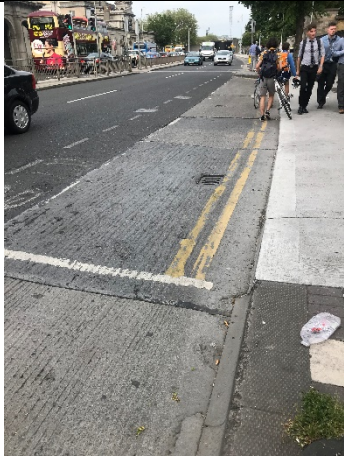
10-09 – Concrete surfacing outside of electrical substation. Concrete appears to be of a different age to surrounding concrete, which could indicate different resurfacing/road works.
