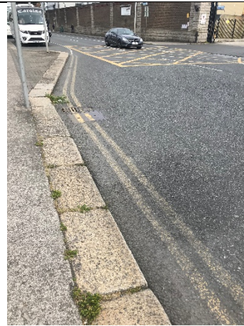
10-06 – Small areas of staining on Victoria Quay consistent with staining from parked vehicles.
