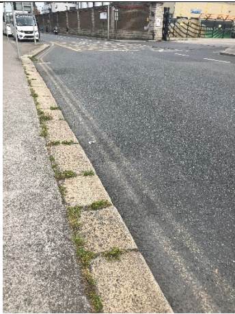
10-05 – Small areas of staining on Victoria Quay consistent with staining from parked vehicles.
