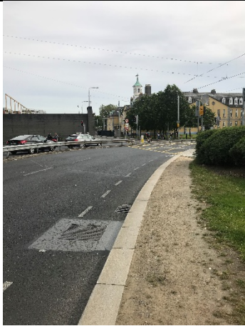
10-01 – Manhole cover observed at indicative leak location, between the road and Luas Stop.
