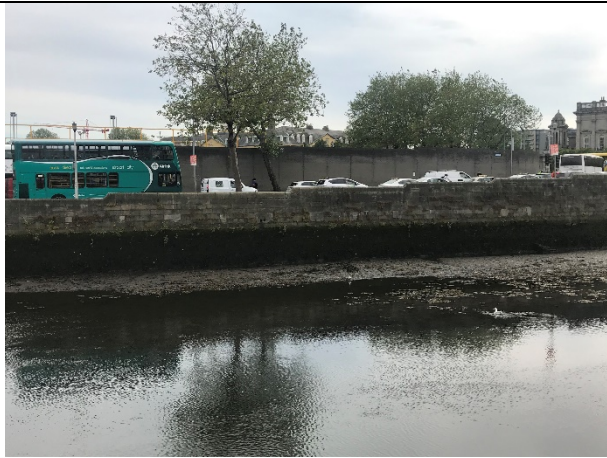
10-03 – Algae, muds, and debris observed on quay wall (observed from opposite side of the river). Appearance on quay wall seems consistent, with little variance or dieback.
