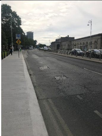
10-07 – Evidence of significant road resurfacing/works in front of HSE building on R148.
