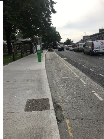
10-08 – Cracks in concrete outside the HSE building on R148 evident.
