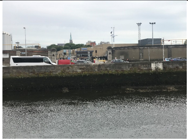
10-02 – Algae, muds, and debris observed on quay wall (observed from opposite side of the river). Appearance on quay wall seems consistent, with little variance or dieback.
