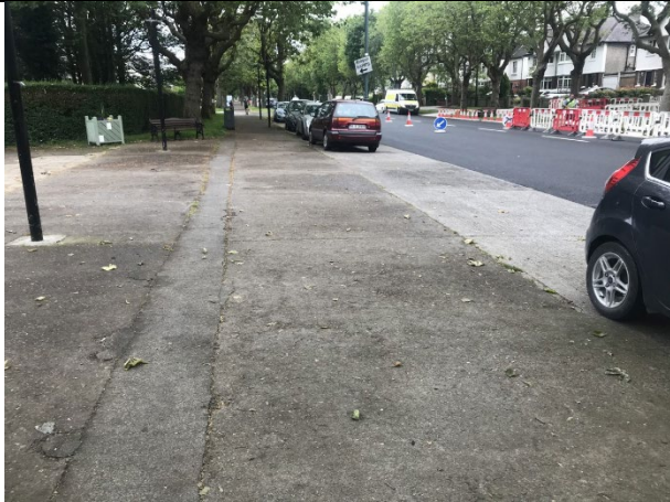
16-01 - No obvious staining on the indicative leak location outside the Corpus Christi Church.
