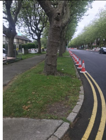
16-02 – Cabling located along footpath/grassed verge, and under concrete section where on-street parking is located outside the Corpus Christi Church.
