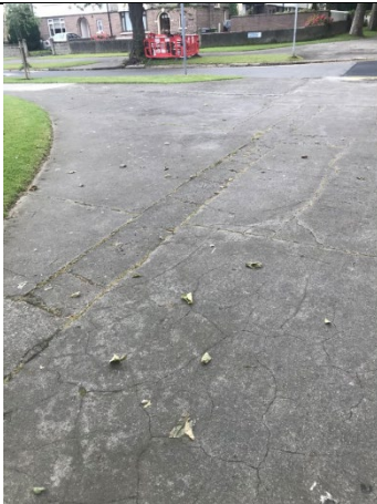
16-03 – Some patchwork noted along the concrete footpath area. Patchwork noted to follow the course of the likely cable at the junction of Clare Road and Griffith Avenue, and outside the Corpus Christi Church. No die back noted on grass.
