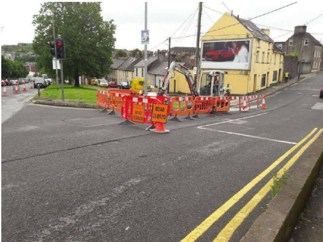
Photo 4 Location of known leak point on eastern side of Wolfe Tone Street. Trial pit works in progress.
