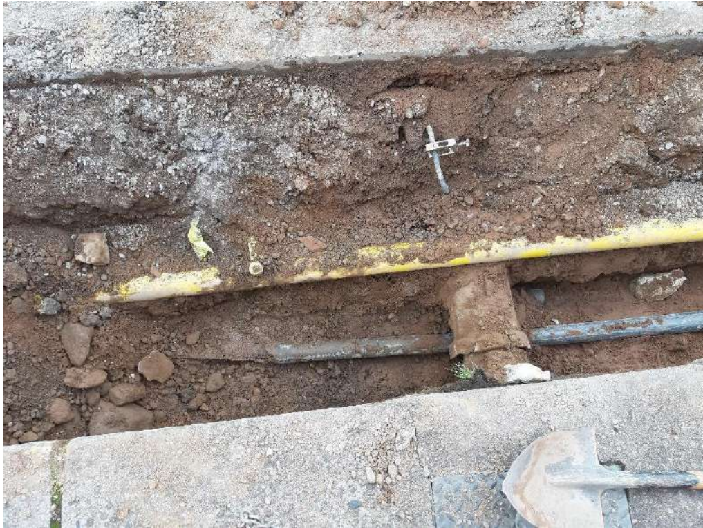
Photo 3 Occurrence of underground services during excavations. Gas, sewerage and communication ducts visible in image.
