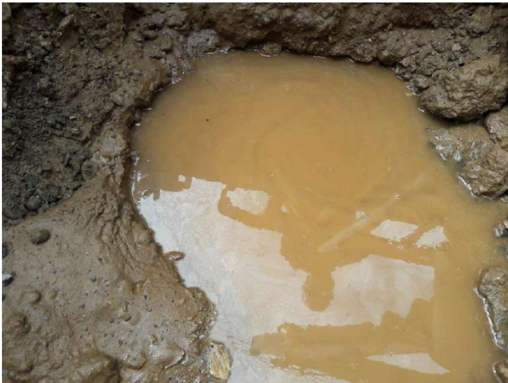
Photo 6. Image showing the ingress of water into trial pit excavation during initial site investigation activities in June 2019. Note the visible hydrocarbon sheen thought to be associated with residual cable fluid in soils.
