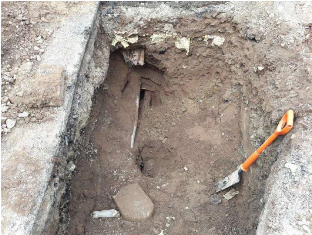
Photo 5 Trial pit and inspection hole works being completed at the location of the known leak point (ESB Ref: 2)
