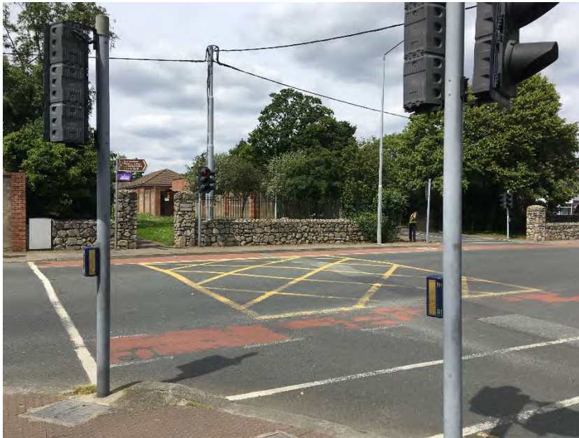
Photograph 1 – Leak location; west side of Brewery Road
