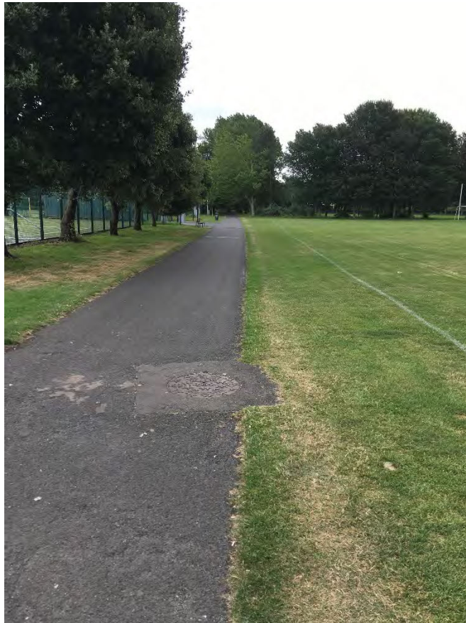
Photograph 1 – View east from leak location
