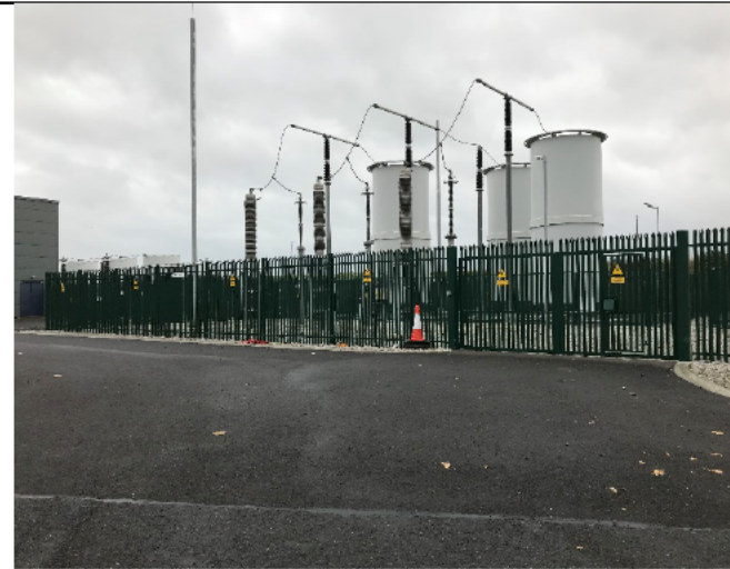
49-05 - No breakout noted along the section at the indicative leak location. However, recent groundworks were evident around the area (new hardcore surface and new tarmac access road). The site representative noted that these works were conducted about 3 years previously.
