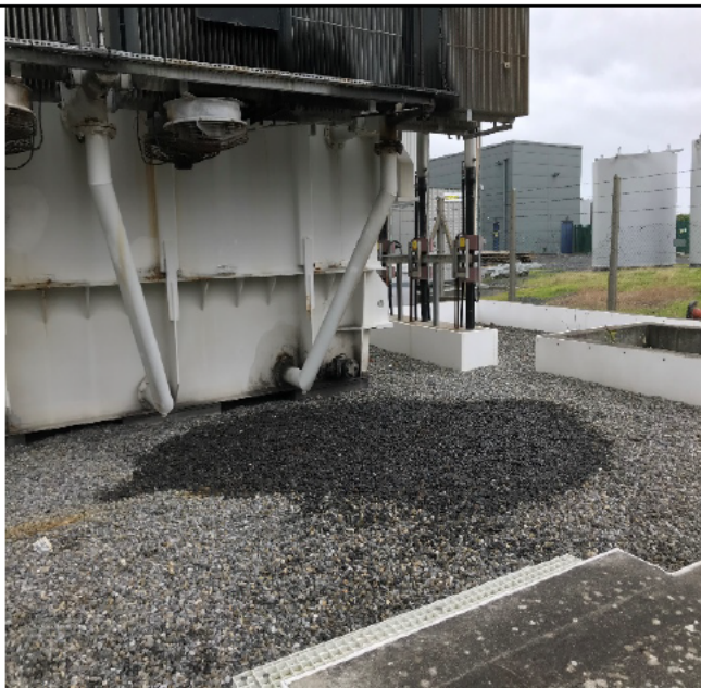
49-03 Staining was noted under the TF4 unit in the bund.
