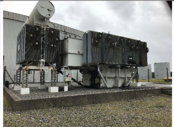
49-02 – the cable route progresses eastward and travels into the compound and to the TF4 transformers. These are positioned over a bund
