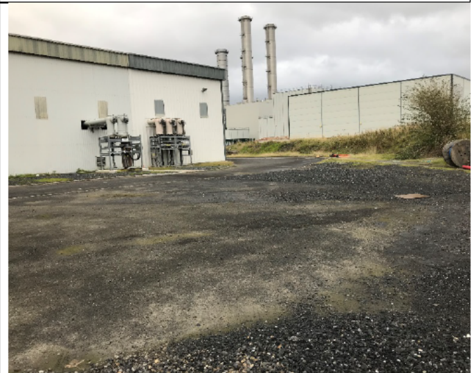
49-08 – One cable (likely removed) travels east and then north and entered the '220 GIS Building'. No overlying evidence of contamination was noted along this route. Break/repairs in the tarmac were noted prior to the cables entering the building
