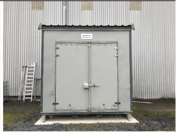
49-06 – A cabin is positioned over the indicative leak location. The cabin was locked but a plate on it's exterior noted 'Carrickmines HV Cable Pressure Tanks'. It is assumed that this may have been built around the time of the other surface works due to the unweather appearance of the concrete under the cabin. There was no staining evident on or around the cabin's base.
