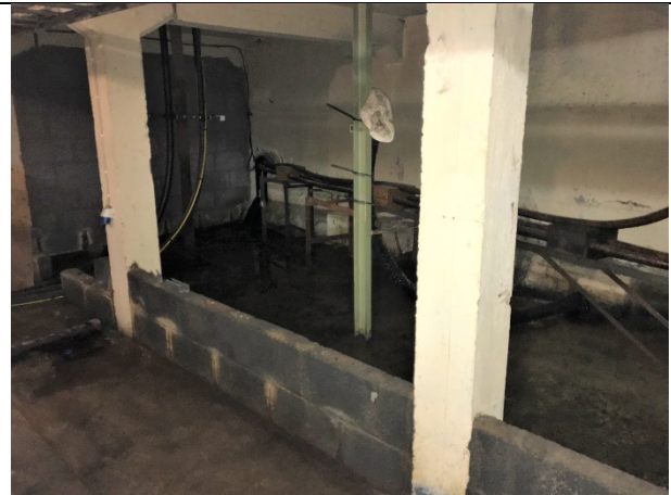
60-08 – A second bund contained a similar amount of liquid build up as the first bund in its base and outside the bund.
