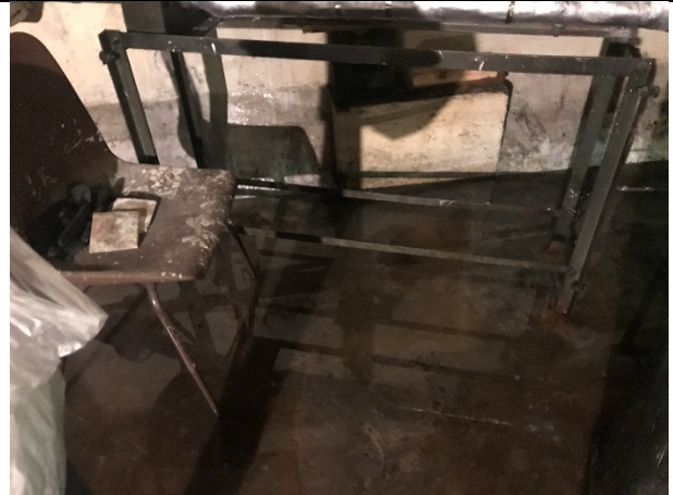
60-06 - Additional staining and liquid in one of the basement bunds.
