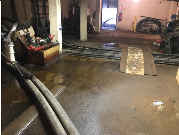
60-05 - Additional staining and liquid in one of the basement bunds.
