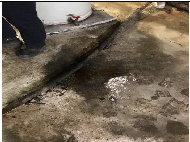
60 -12 – Additional oily staining within the substation basement.
