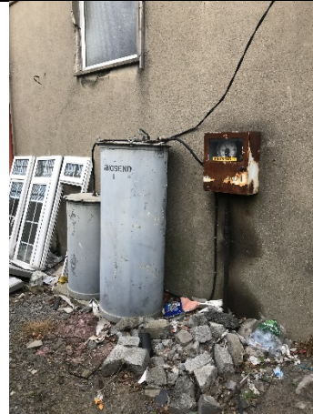
60 –14 – A fill point similar to the tanks in the first basement bund was found externally on the northeast corner of the substation building. Staining was not noted on the external sides of the tanks or on the hardcore surface, however staining was evident on the pipework and the wall behind the pressure valves.
