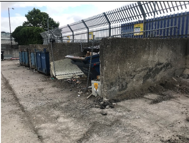
60–15 – From the mapping it appears that the section of interest runs northwards within the ESB networks property, under a waste storage area. This area has a patched concrete base.
