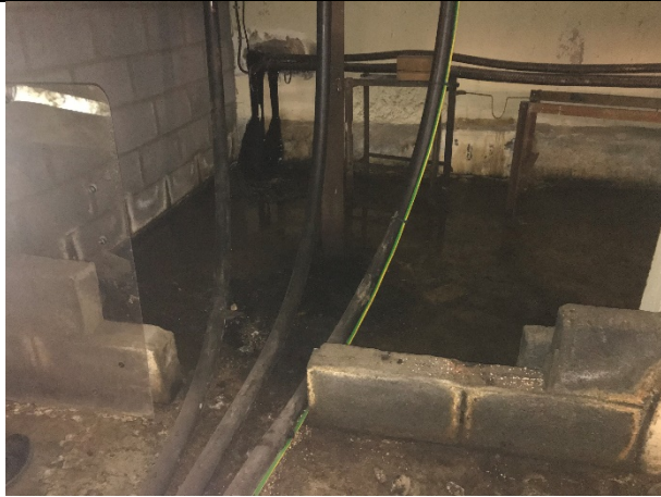
60 -09 – The perimeter blocks of this bund had been removed in one area to accommodate three cable lines.
