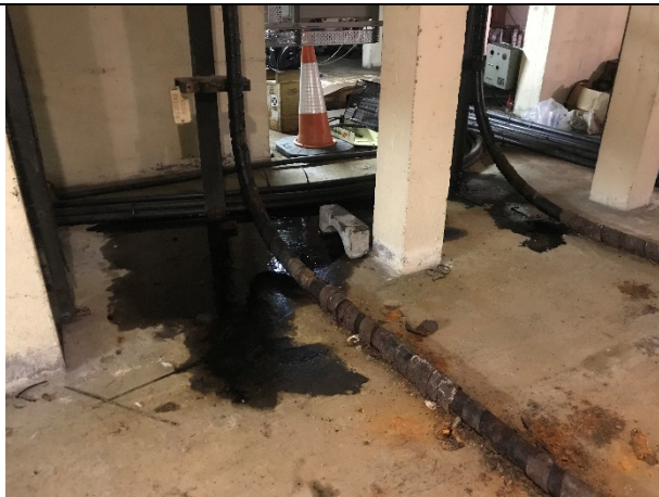
60 -11 – Oily staining was noted in several other areas within the substation basement. Some staining was noted by the site representative to be bitumen, which was previously used as a type of insulation.
