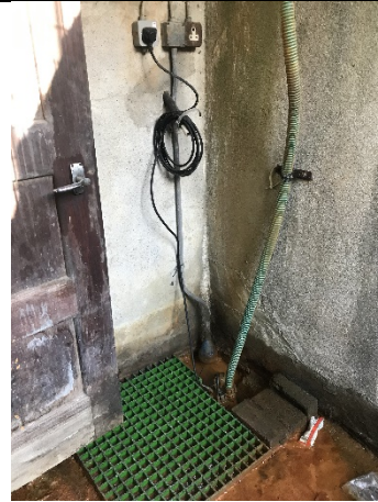
60 -10 – A further sump and pump were noted in another stairwell into the basement (northern side of the building). The sump contained a red rusty residue
