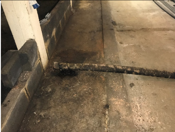
60 –13 – Additional oily staining within the substation basement.
