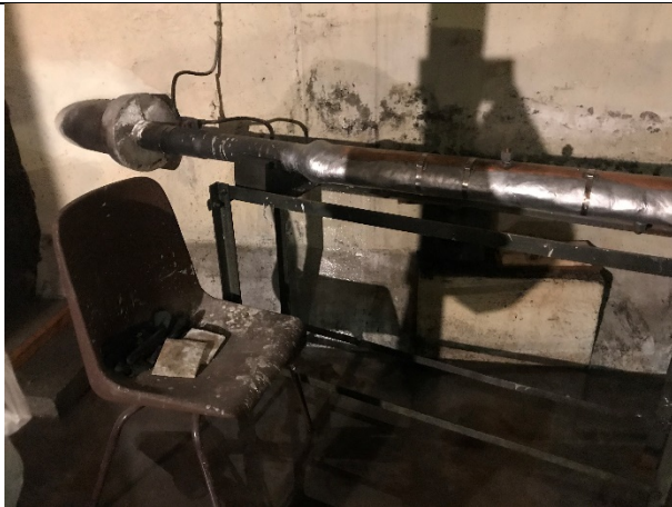
60-07 – Oily staining was noted on the wall to the rear of the first bund.
