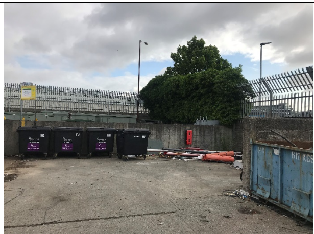
60 –16 – Additional patched concrete base under a waste storage area.
