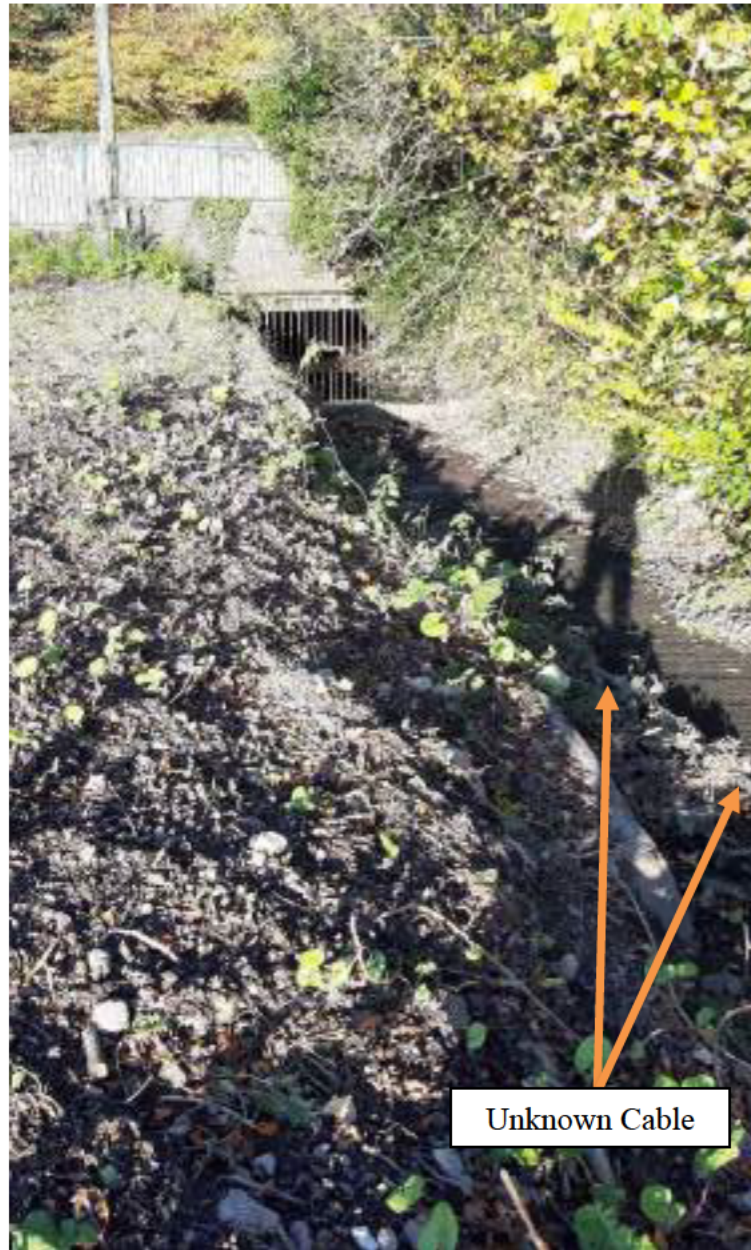
Photo 3. Photo looking north from Glasheen River park area, towards Glasheen Bridge and cable leak point. Note the small concrete weir (dry) and debris at entrance to bridge. Near-stagnant flow. A 2-3" diameter pipe/cable of unknown purpose was seen to follow River and pass under the bridge.
