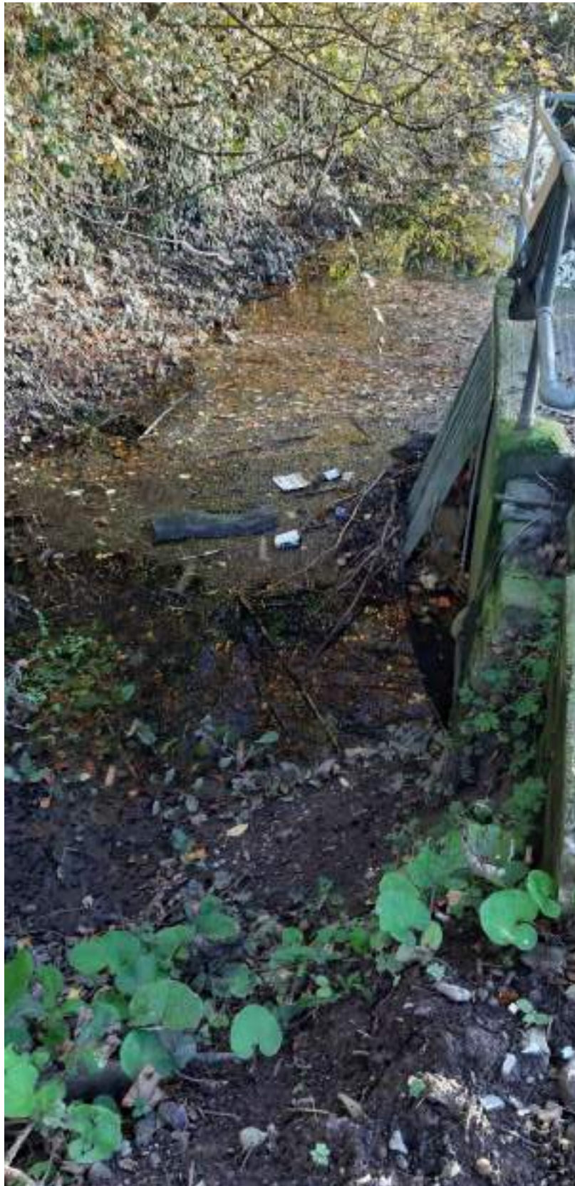
Photo 4. View, looking south, of Glasheen River (35m from leak point) showing the location of the diverted channel of the River and associated diversion/treatment/pumping channel and grate. Note that the bulk of flow on the river was flowing into this grate.
