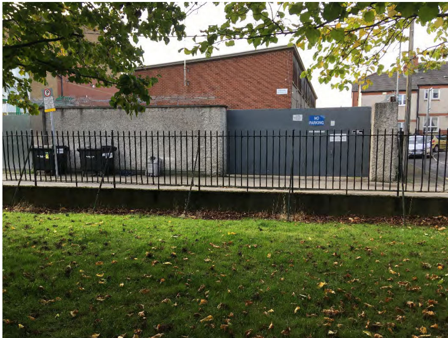
Photograph 4 – 38 kV substation west of leak location
