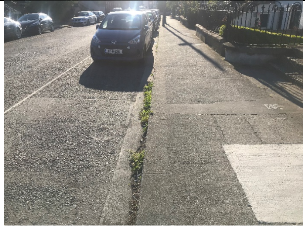
7-14 – Numerous water connections perpendicularly crossing the section of interest on Pleasants Street. Repaired sections lead to water meter covers.
