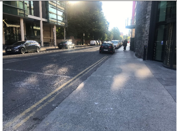
7-06 – Road surfacing in good condition on Hatch Street Upper. Staining noted on surface, typical of minor losses from parked cars.
