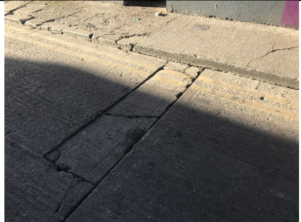
7-10 - Numerous sections cut from concrete on Camden Place. Indicative of repairs or access to subsurface utilities.
