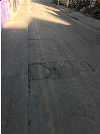
7-09 – Numerous sections cut from concrete on Camden Place. Indicative of repairs or access to subsurface utilities.
