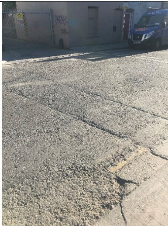
7-11 – Road surfacing in good condition on Pleasants Street. Some sections of previous works evident, indicative of repairs or access to subsurface infrastructures.
