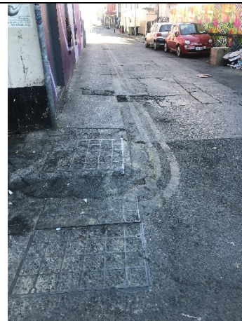
7-08 – Staining noted along section of interest (approx. 25 m west of indicative leak location, on Camden Place); however, appears consistent with bins stored locally.
