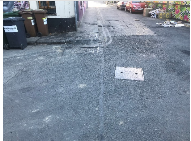
7-04 – Camden Road surfacing is a mixture of concrete and asphalt. The concrete surface was noted to be damaged in several areas and HGV movements were noted on Camden Place.
