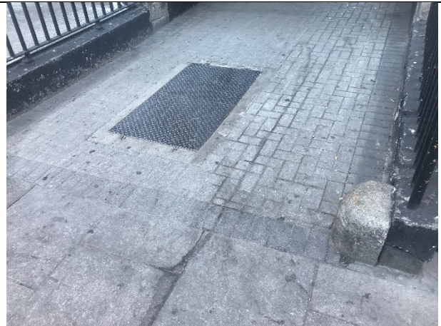
7-02 – Staining noted on footpath surface at indicative leak location. Consistent with surrounding staining, likely resulting from activities associated with the adjacent nightclub.
