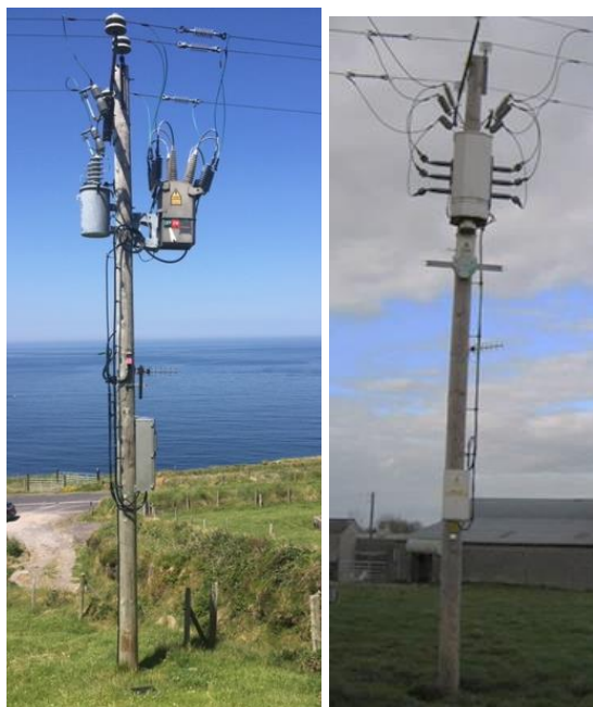
Figure 5.6 Network automation equipment
