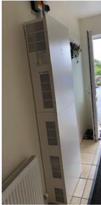
FIGURE 4 - SONNEN BATTERY INSTALLED AT TRIAL PARTICIPANT PREMISES
